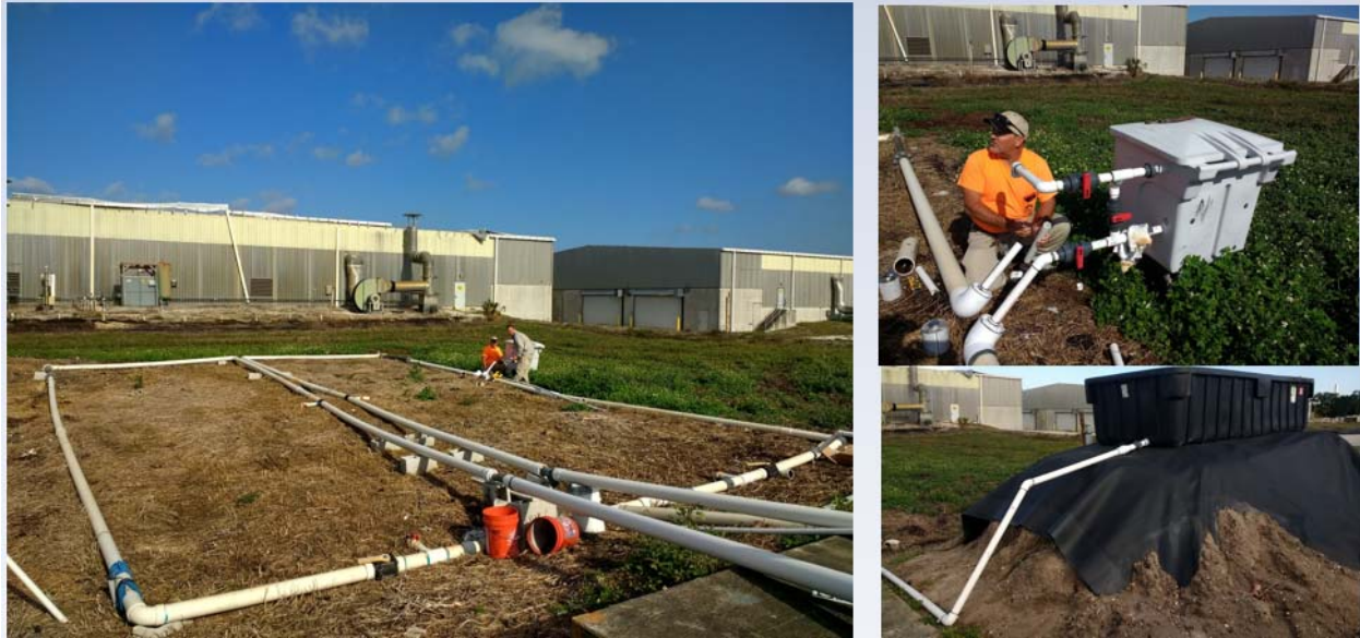
Figure 2. Field scale pipe network at the landfill (left), UV unit installation (right top), leachate storage unit (right bottom)
